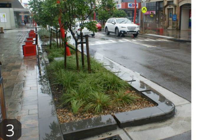
3 Rain Gardens between parking bays collect overland flow through slotted kerbs, filtering it to improve stormwater quality prior to being piped to the existing pond
